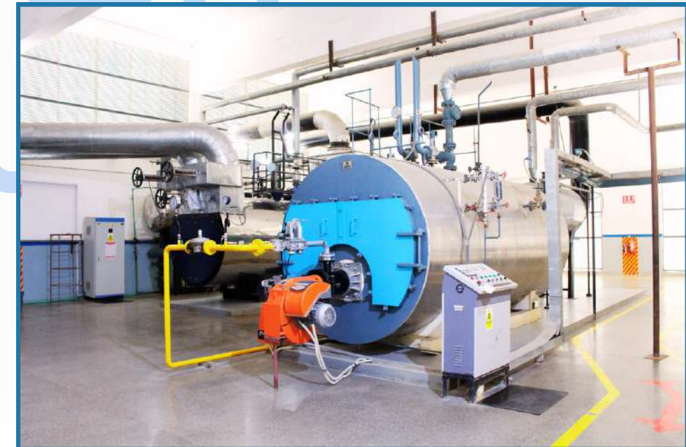
Gas fired boiler 4 Ton
