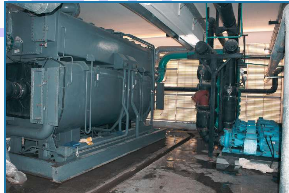
Absorption Chiller 360 USRT
