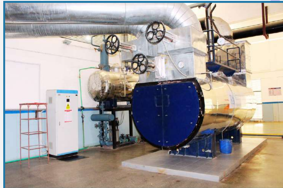
Waste heat recovery Boiler (WHRB) 1700 KG
