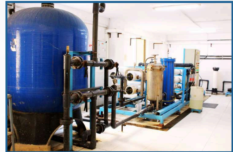
RO plant 120,000 gallon/day
