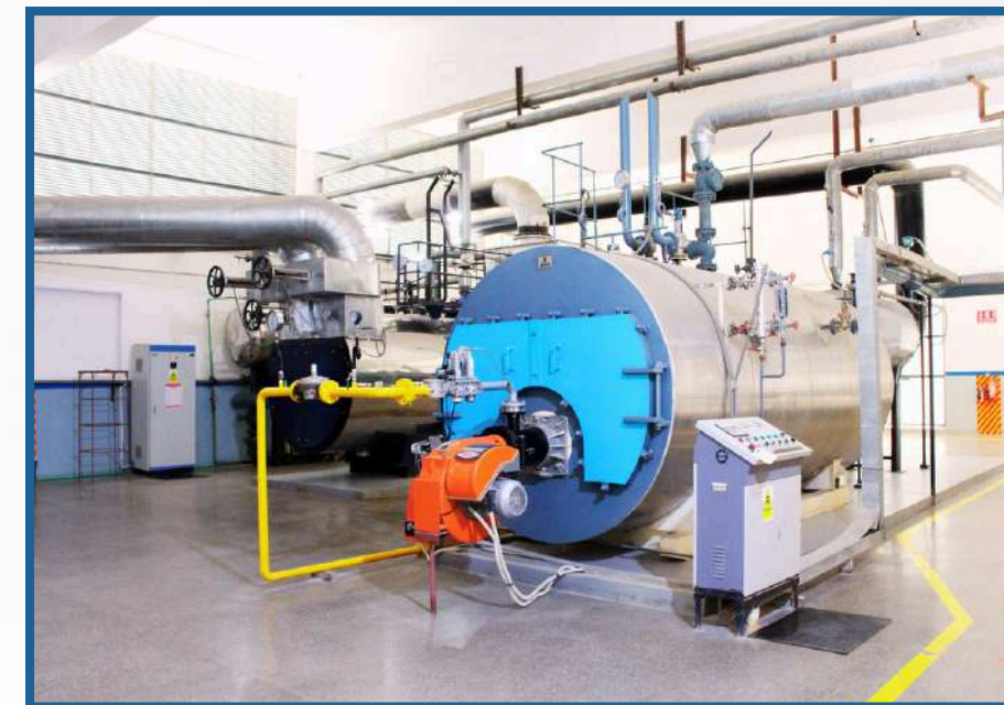
Gas fired boiler 4 Ton
