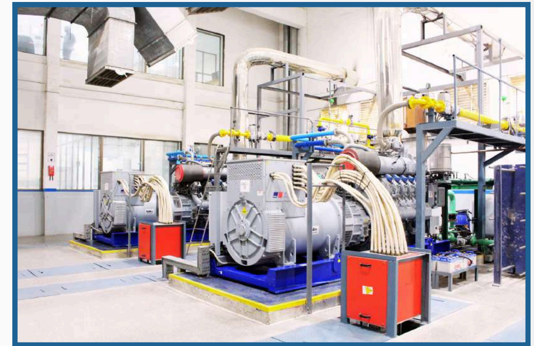
MTU 12V 40L64 Gas Generator (1521 KW)
